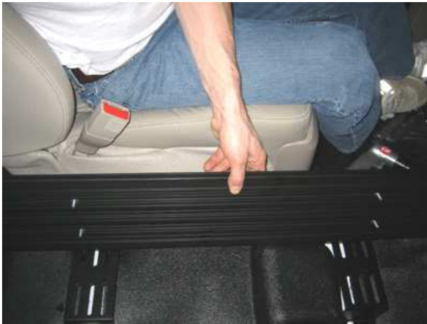
Position the nuts to line up with the slots in the C-B10 brackets previously installed.
