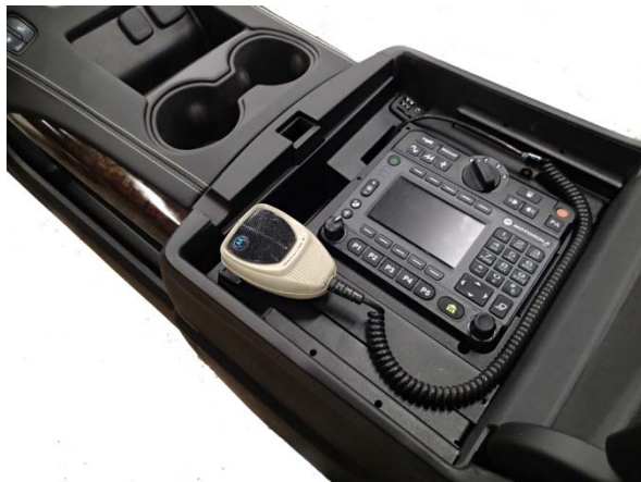
Driver side view with another control head and microphone. Make sure mic is located so arm rest lid can close properly
