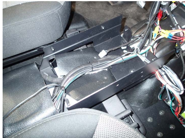
Carefully place and bolt front hump bracket to floor with previously removed OEM floor bolts. Wire harnesses go on top of bracket. Note: Rubber mat will need to be cut first.
