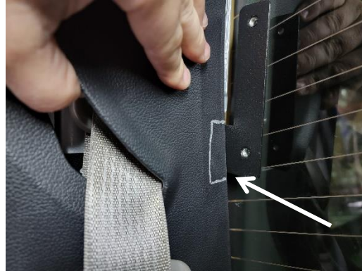
Mark section of trim to be notched to allow clearance for bracket.
